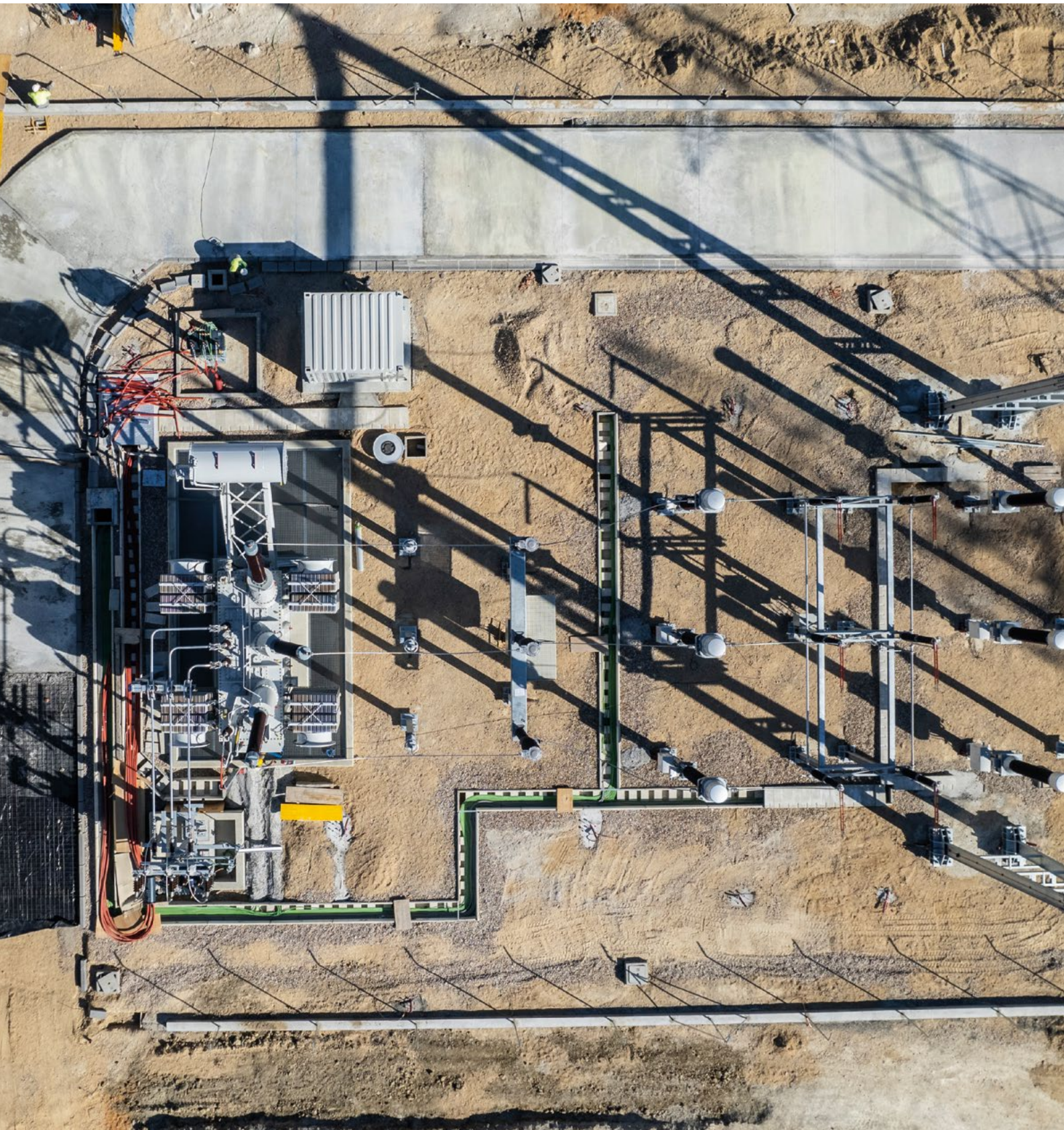
A substation was built for the Spanish wind farm Andella in the autonomous community of Castile and León, which was commissioned in June 2024.
