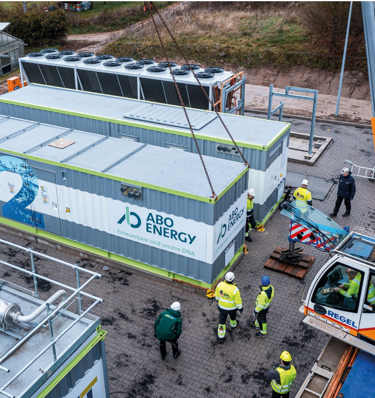
In November 2024 the electrolysis containers were delivered to the project in Hünfeld-Michelsrombach.
