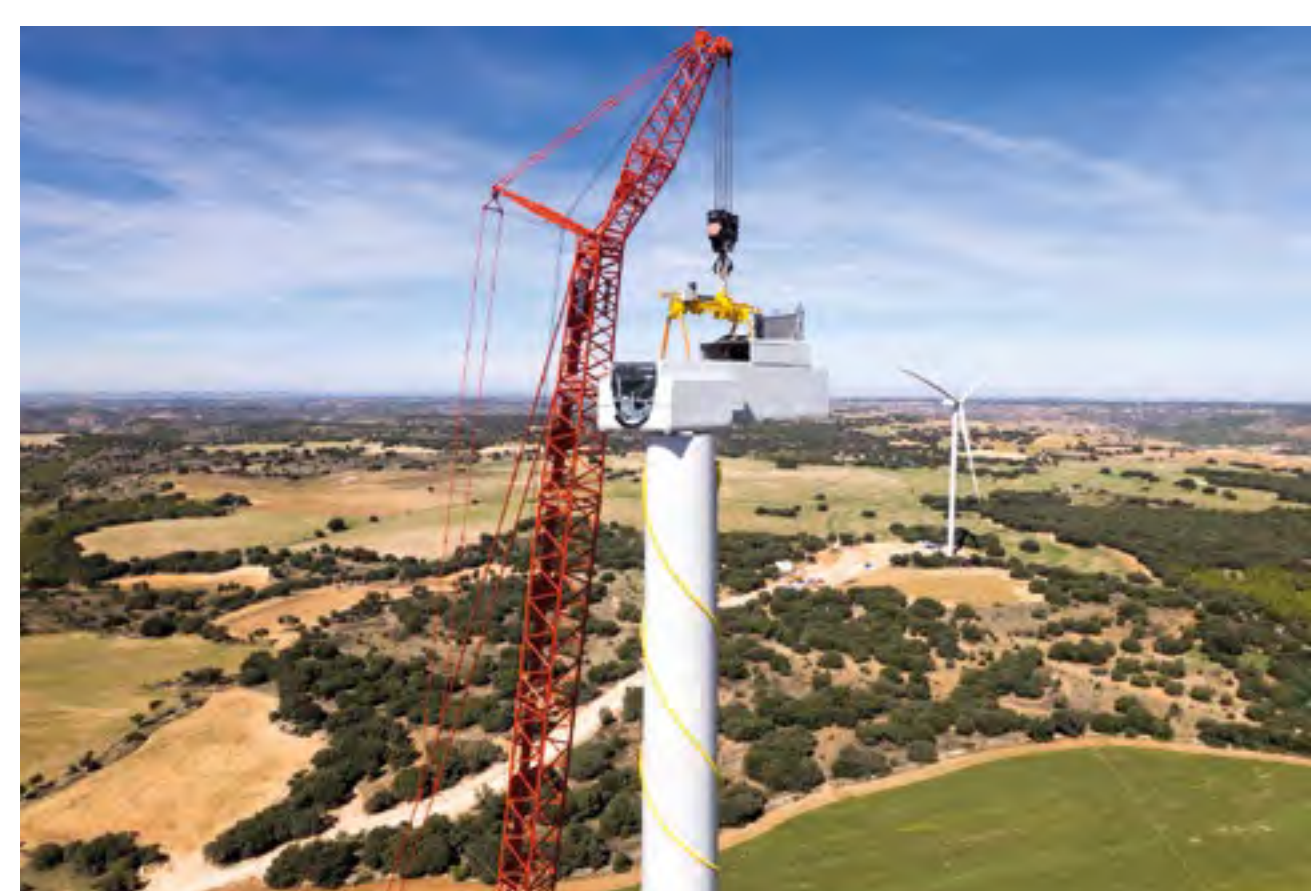
Once the tower has been erected, the gondola is placed on top
