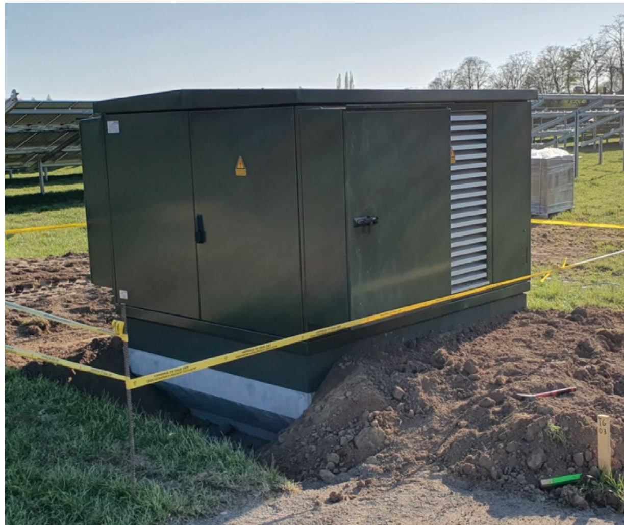
Trafostation (PV-Anlage Kevelaer; 2020)
